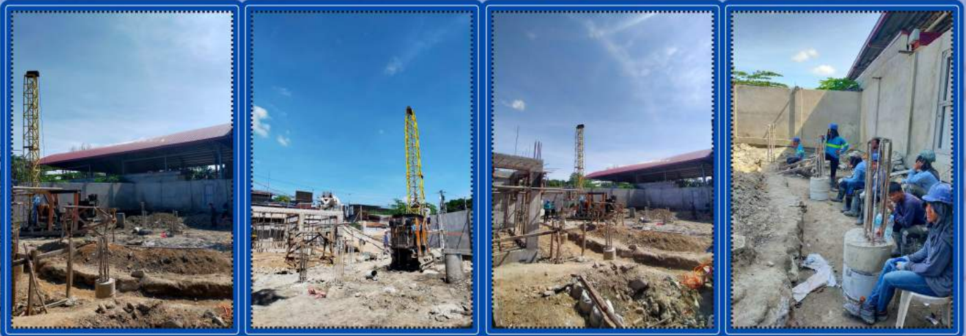
Concrete pouring of bored pile 17/17 at Banga 1st also part of Ground reservoir project
