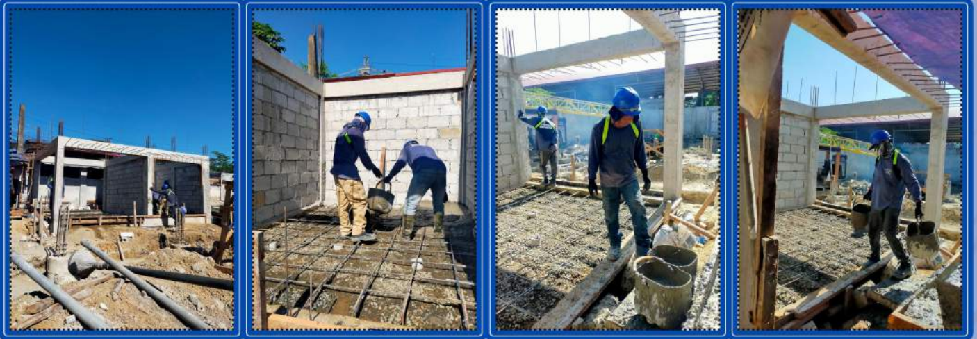
On going construction of pump house at Banga 1st part of 1,500cu.m. Ground reservoir project
