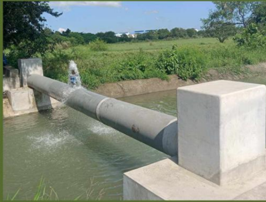
Energization of IP-2 an additional water supply for Brgy. Banga 1st, Banga 2nd and Bagong Silang
