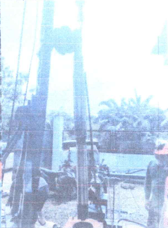
New Pump and Motor.
